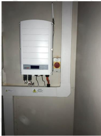
Figure 4: SolarEdge inverter with WiFi module for monitoring
